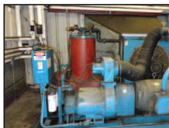
One of (3) Quincy 200hp & 300hp Rotary Air Compressors
