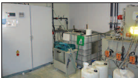
Tecnotrans Nickel Waste Treatment
