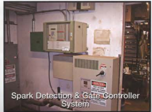
Cyclone Dust Collection System
