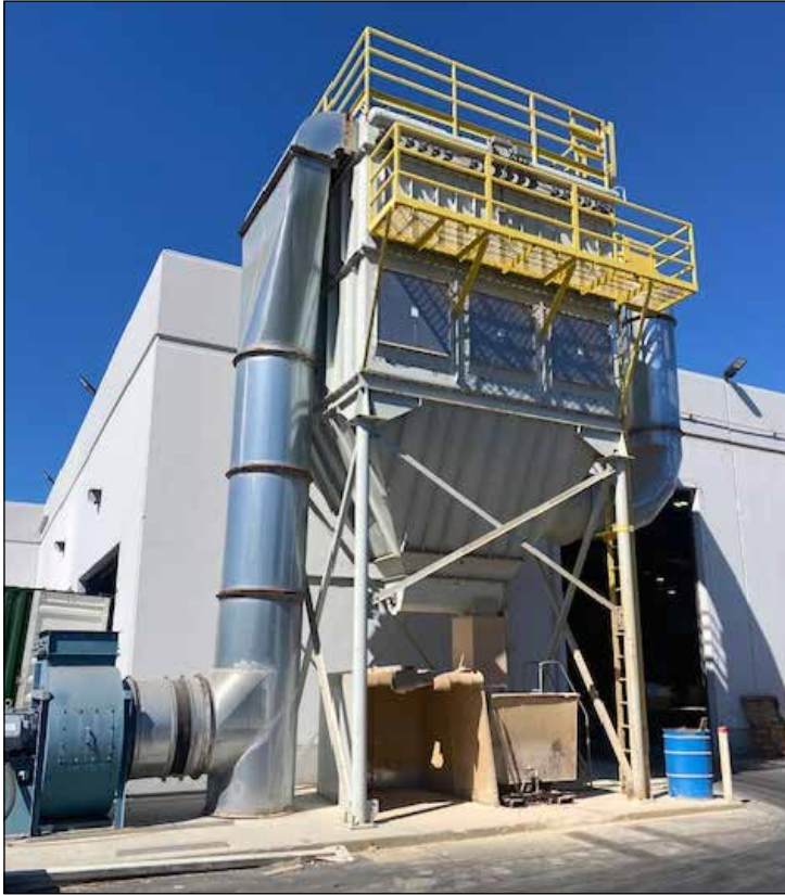
Torit Donaldson Dust Collection, w/Twin City Mod. BCS-SW
