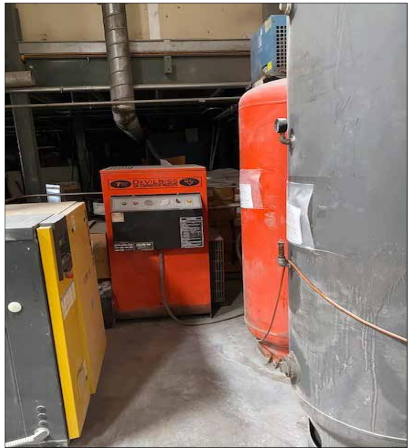
View of Air Compressors
