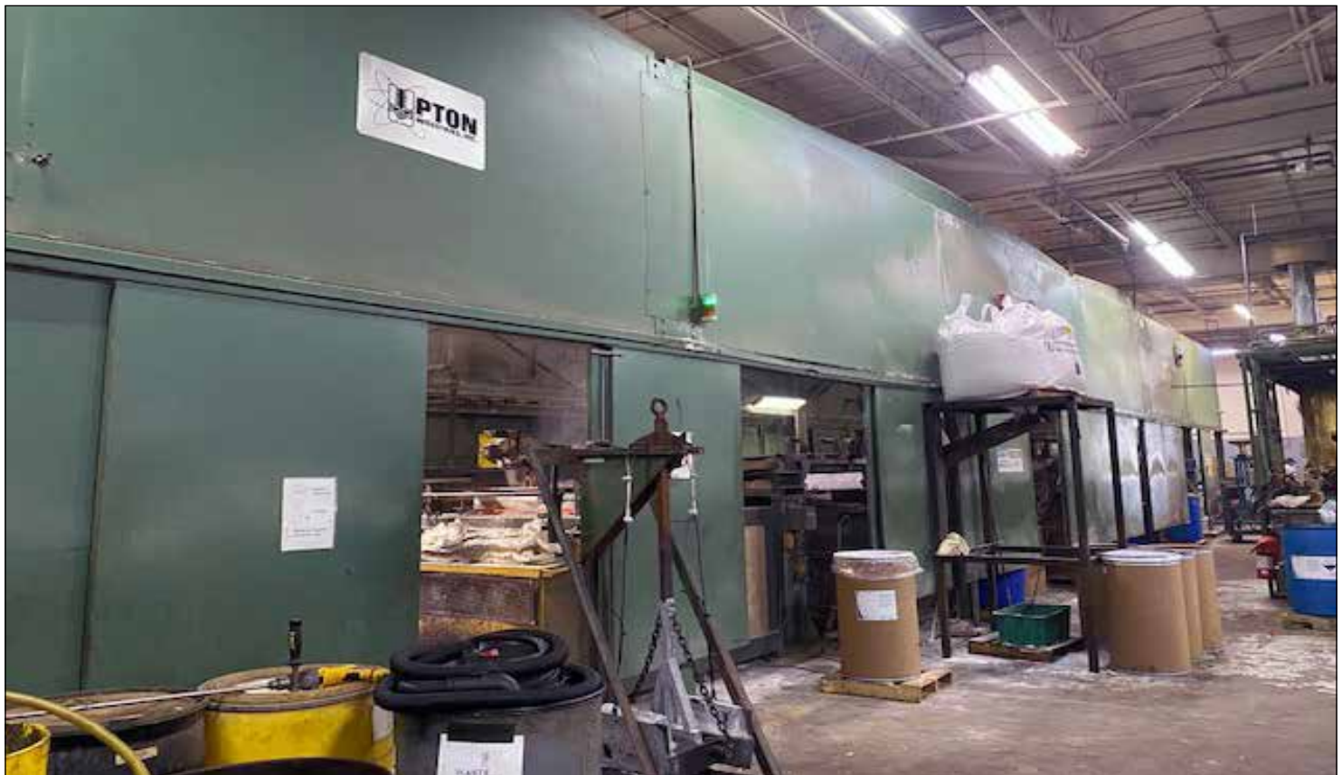
View of Upton Heat Treat System
