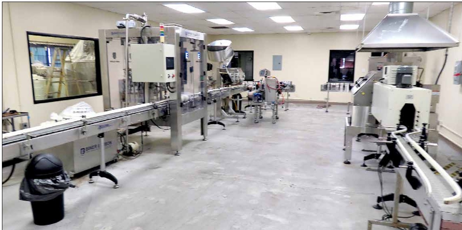
Rotary Liquid Filling Line
