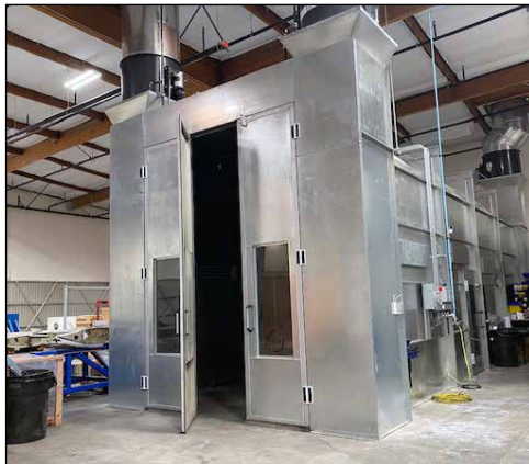
RGI Sanding / Paint Booth
