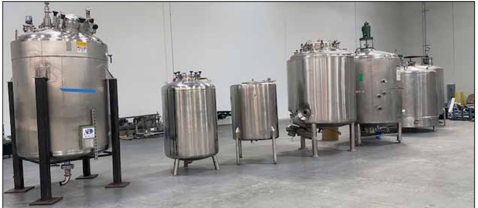
Partial View of Tanks
