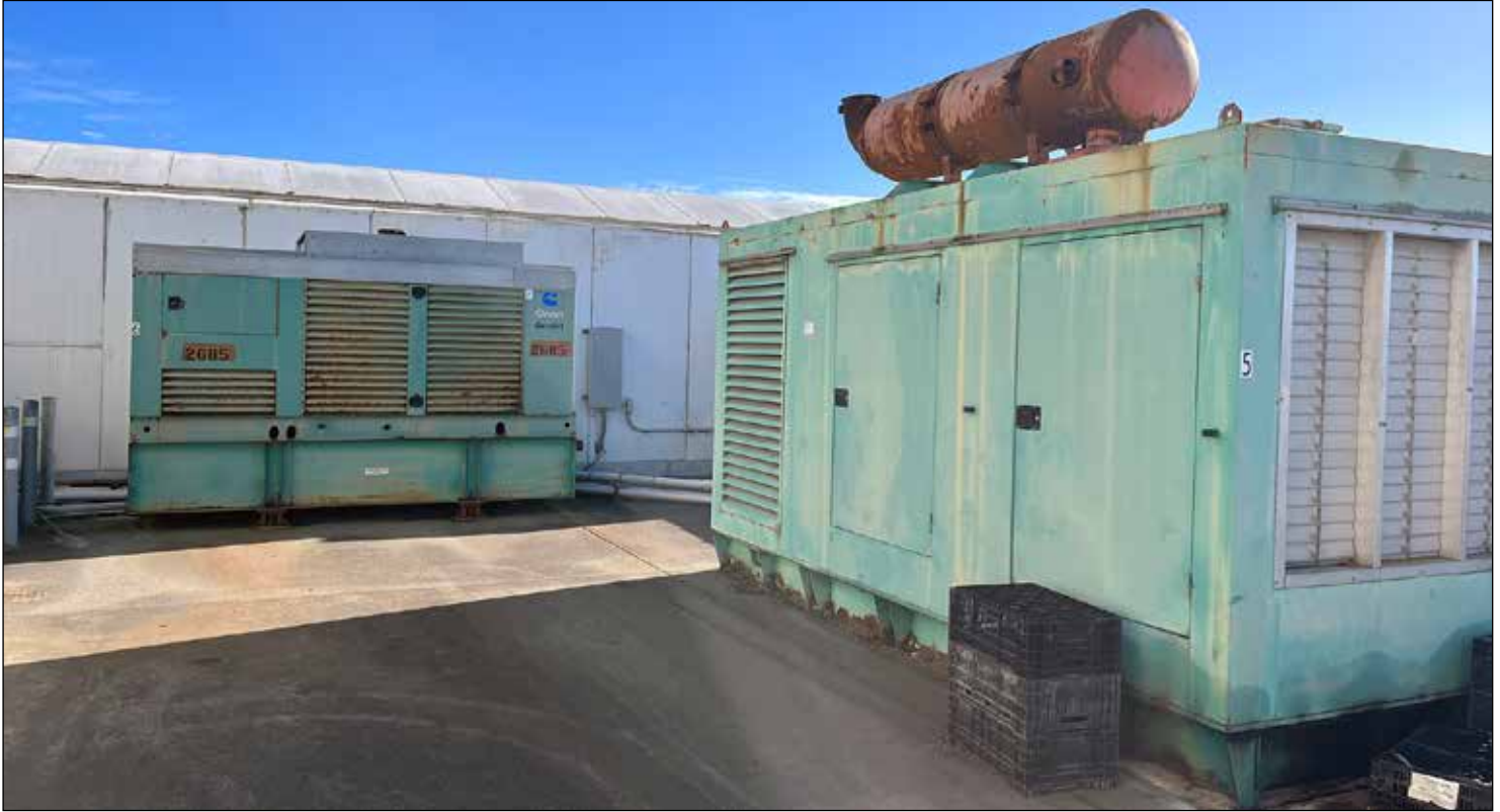
Onan Mod. DFRH-5002064 400-KW Generator
