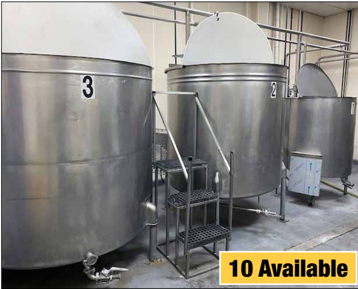
Partial View of S.S. Mixing Tanks
