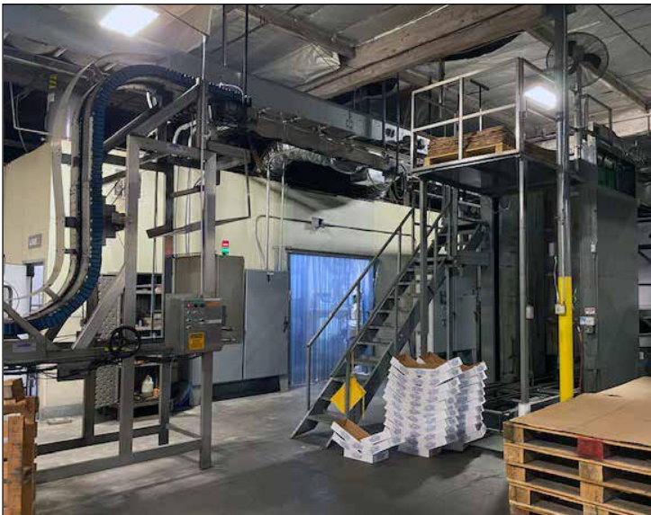
Seco Mod. 300-20 Palletizer, w/Ambec Conveyor System
