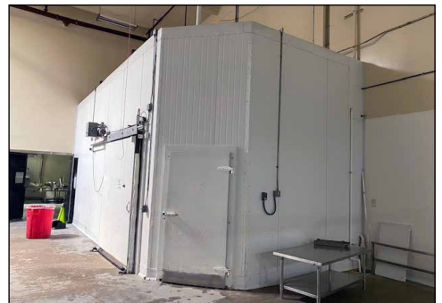
30' x 15' Cooler Room
