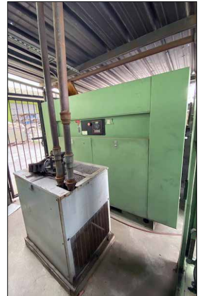
Sullair Rotary Screw Type Air Compressor
