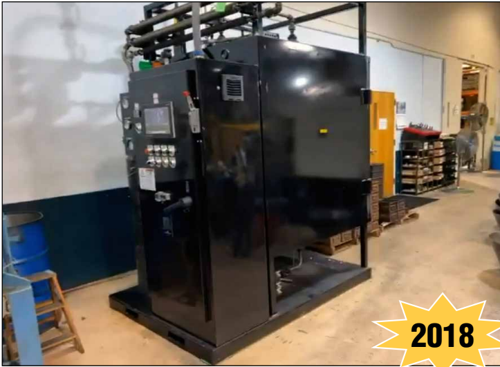
Atmosphere Engineering A11879 DA Generator
