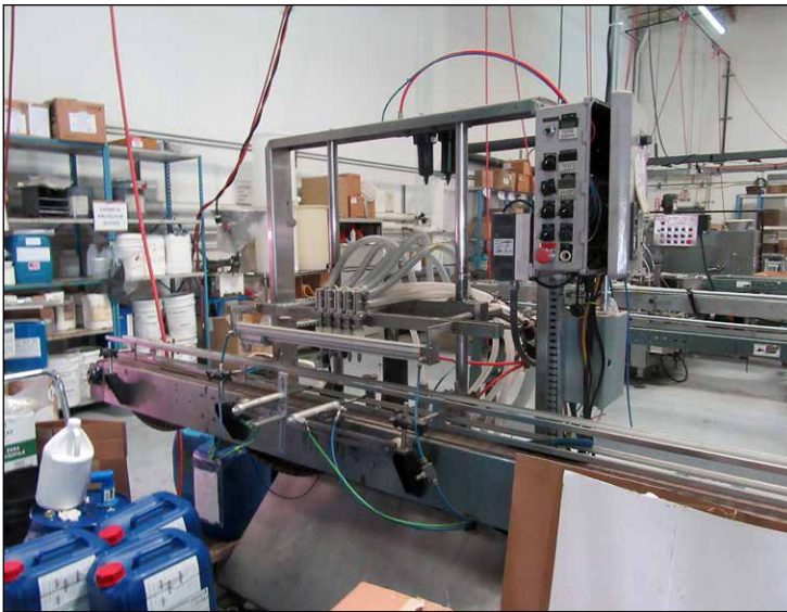
5-Station Filling Line
