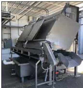
Waste Water Hydro Sieve
