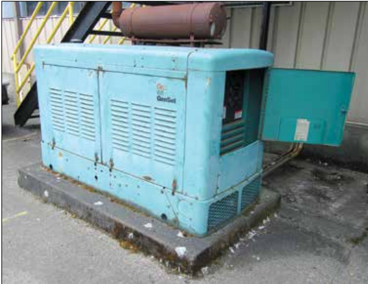
Onan Mdl. 45EM L33757R Natural Gas Generator Set
