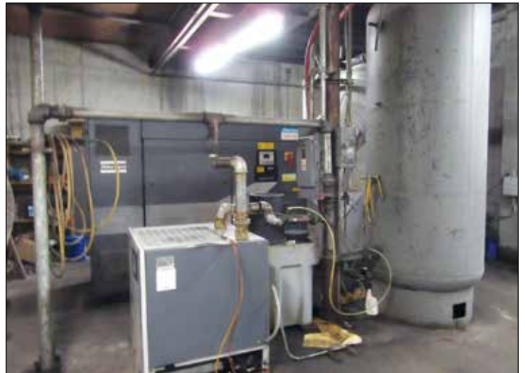
Atlas Copco Mdl. GA90VSD Rotary Screw Air Compressor
