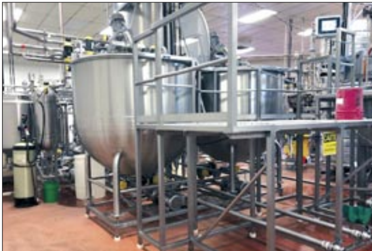
Aseptic Filling Line: Tube-In-Tube Heat Exchanger
