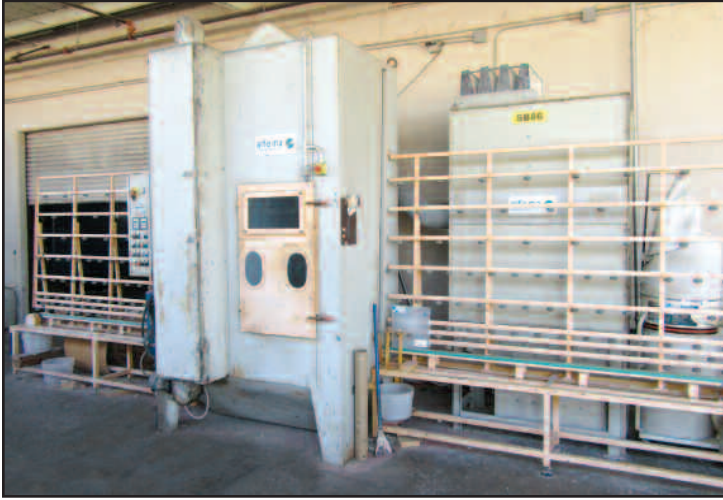
Alfema Glass Sand Booth w/Dust Collector
