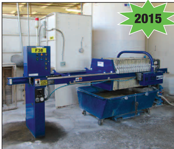
Waste Water Treatment System w/J-Press
