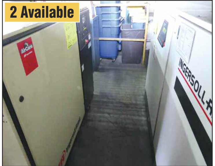
Ingersoll-Rand 60HP Rotary Screw Air Compressor
