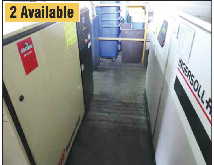
Ingersoll-Rand 60HP Rotary Screw Air Compressor
