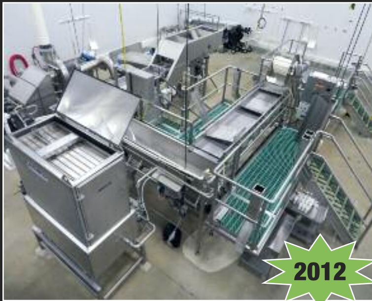
Overall View of Fresh Pack Processing Line
