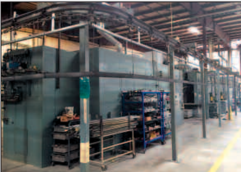
Overall View of Powdercoat Clean & Spray Line
