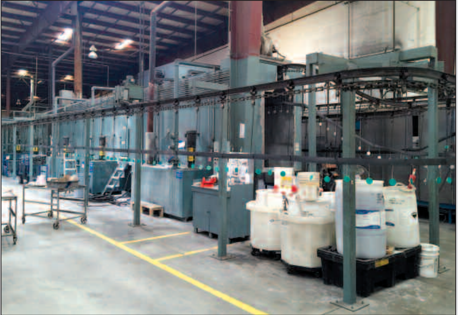
Overall View of Powdercoat Clean & Spray Line
