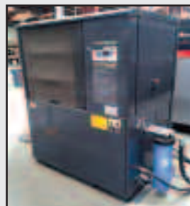
Orion Inverter Chiller
