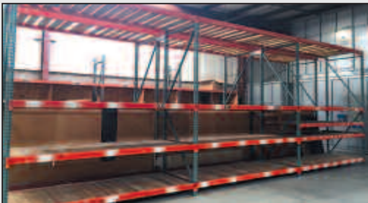
Partial View of (175) Section of Pallet Racking
