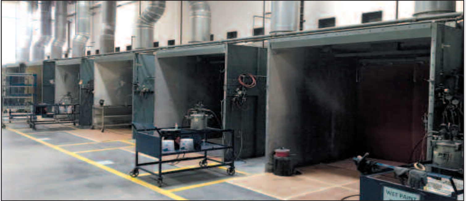
Overall View of Paint Booths
