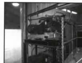
(2) Kaeser N501G, 25hp Air Compressors
