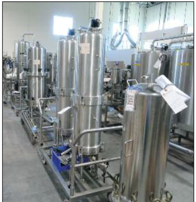
View of Filters
