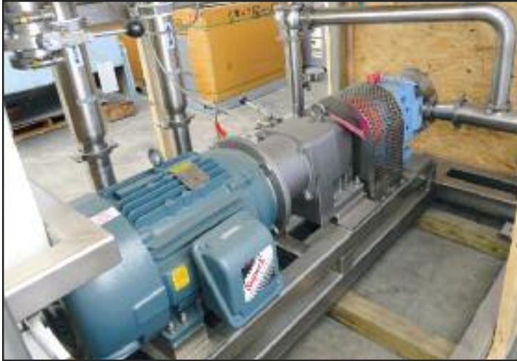
Waukesha 25hp S.S. Pump
