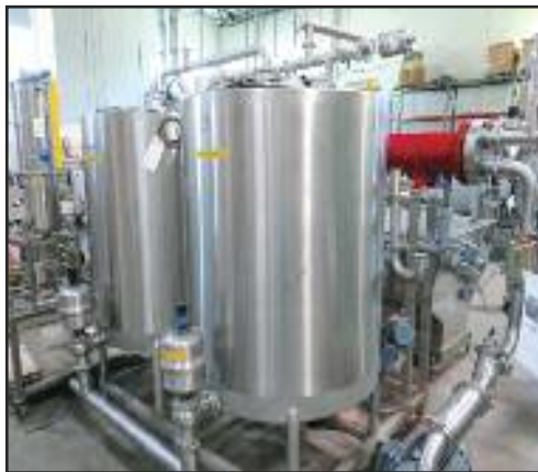
APV C.I.P. System w/(2) 400 Gal. Tanks
