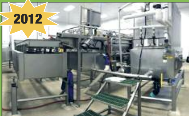
NSEP Cold Water Rinse Line with Mueller Chiller
